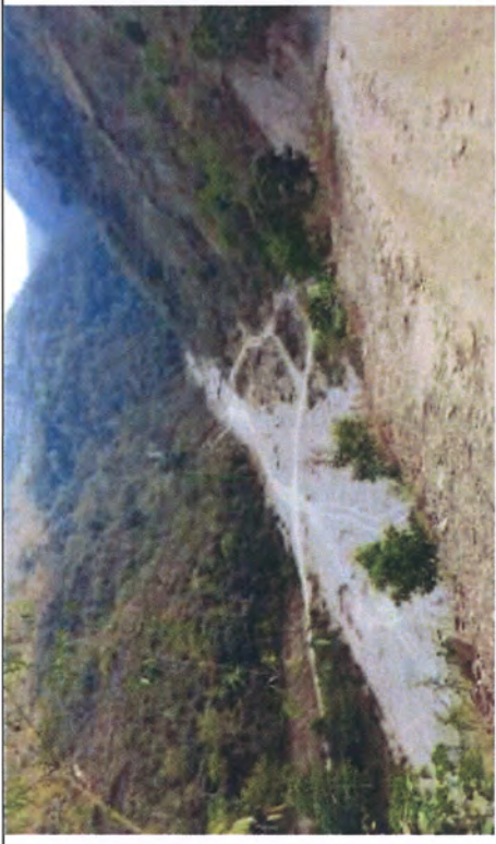
Photograph 13 Khaharekhola at chainage 16+560 further investigation recommended
