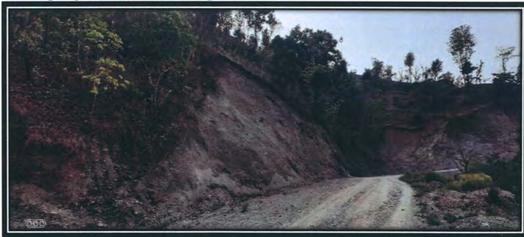
PHOTOGRAPH 3 STEEP CUTTING ON SLOPE OBSERVED AT 16+000
